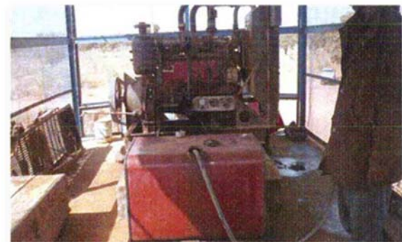
5. Disorder in the pumping station.
