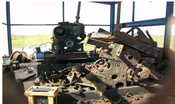
6. Mobile pumping station not functioning.
