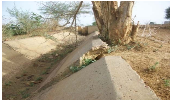
2. Canal panel (first area) detached.
